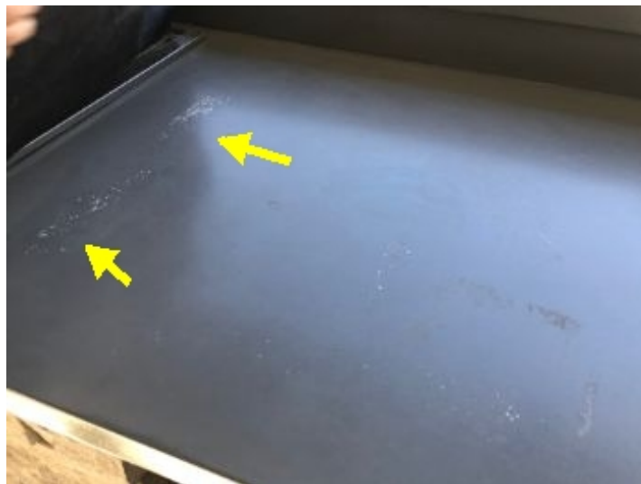
Cement counter top stain/paint is peeling from surface.
