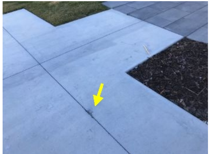
Cracking/Chipped areas observed at the concrete surfaces. Further deterioration will occur as water expands and contracts from freeze and thaw cycles. Recommend sealing the cracks to prolong the life of the concrete.
