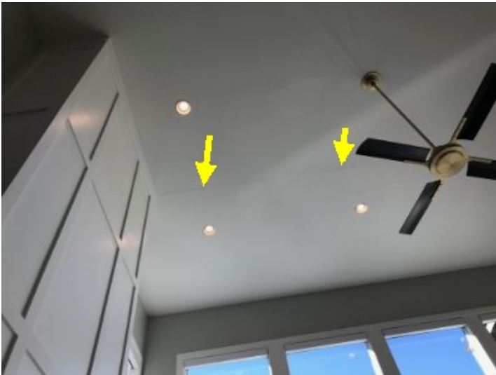
Ceiling cracks observed at sheetrock seams, new construction settling.
