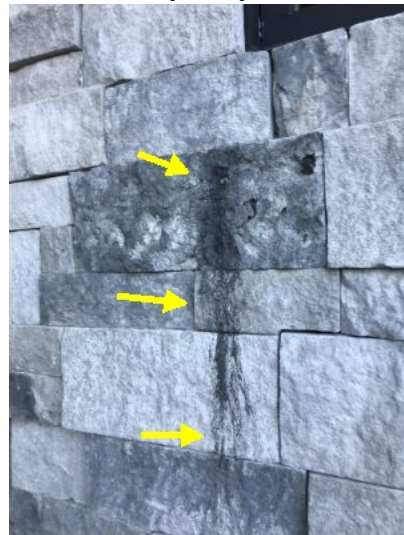
Several deteriorated stones on siding and mailbox. Eroding in place.
