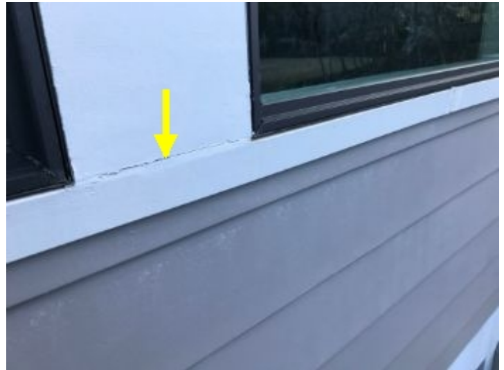
Caulk and seal all gaps, cracks and openings as part of routine yearly maintenance.
