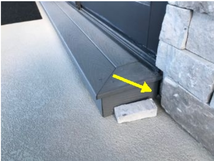
Several loose stones on siding.
