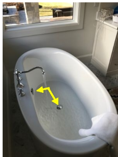
Master bath Stopper and vent is loose/inoperable.
