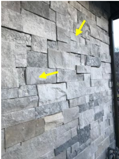
Several loose stones on siding.
