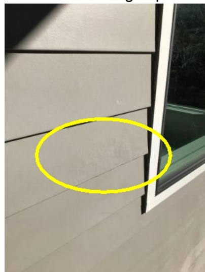
Defective section of hardi-board siding on SW corner by master patio.
