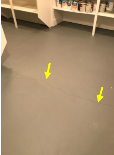
Common cracks noted.
